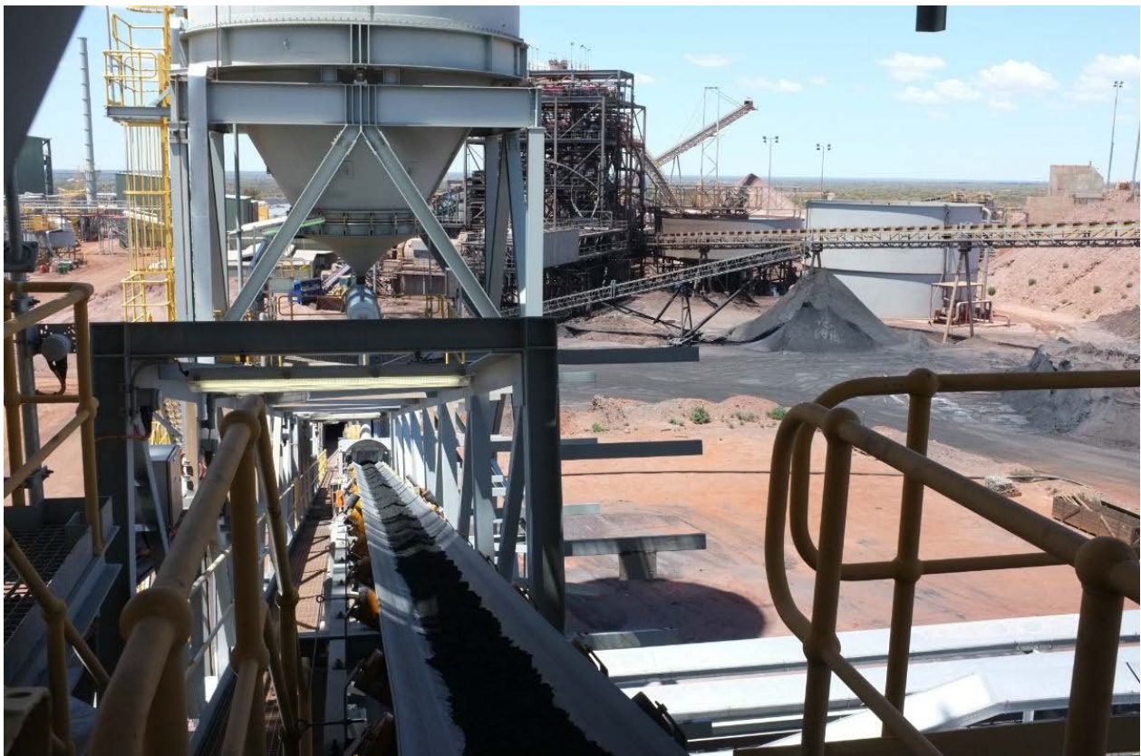
Magnetite concentrate on a conveyor to the kiln at Windimurra
